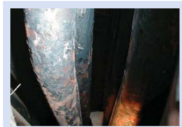
Figure 9: Tubing Exfoliation Caused by Slagging/ Plugging and Poor Gas Distribution
