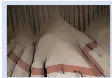
Figure 10: Effect of Ash Plugging on Gas Flow
